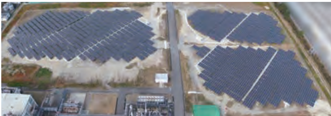
Onahama Plant: the onsite solar power system
